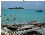
Destroyed berth, Gosier
